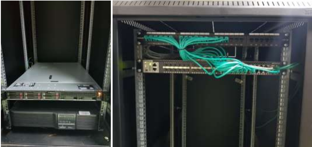
Fig. 9 Communication equipment in the rack
